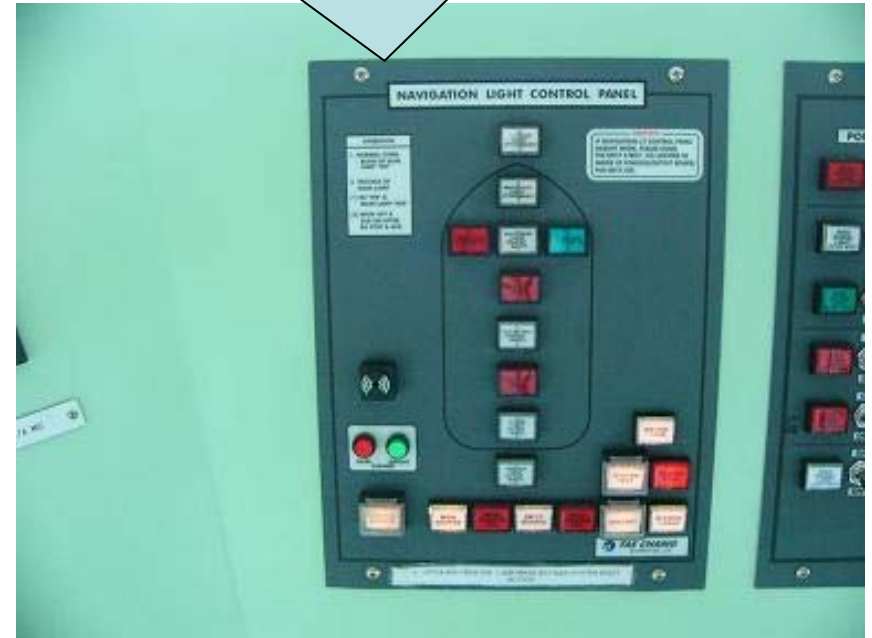
Naviagtion Lights control panel
