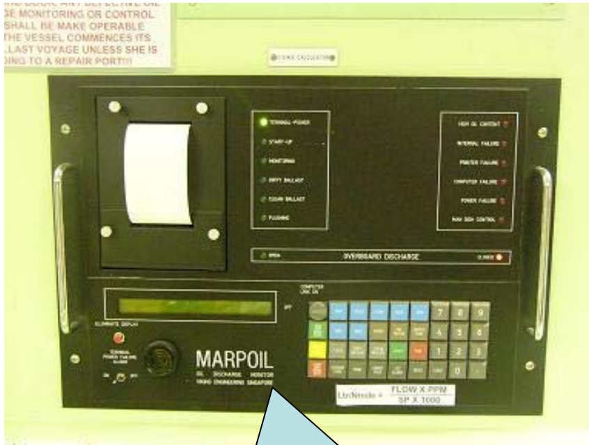
Oil Monitoring Control Equipment panel
